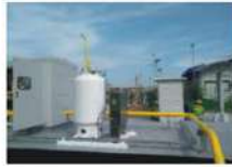
Odorizer Injection System
